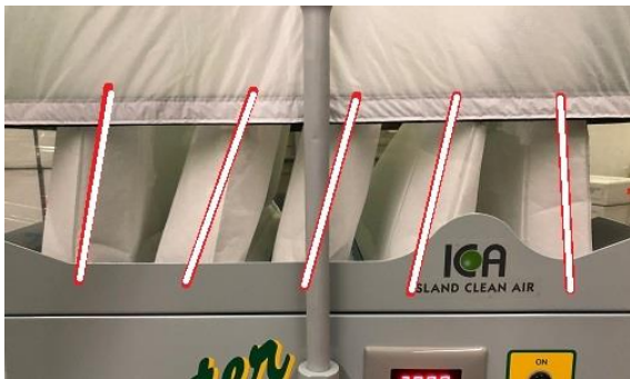
Bent & Not Aligned
